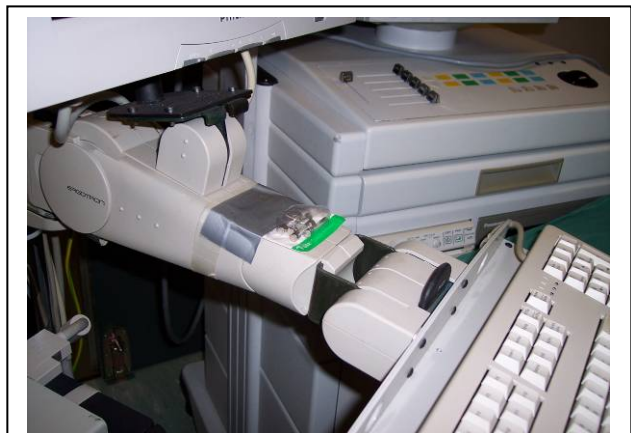
Fig. 2: Example of "tape analysis". Shown is an OEM supplied trolley, which by itself fulfilled all requirements of IEC 60601. Violating this standard, the trolley was retrofitted with equipment drawing more power than the built-in safety transformer was specified for. Therefore the built-in fuses sometimes blew. Following the principle of Le Châtelier & Van't Hoff, someone "solved" the problem by taping spare fuses to the keyboard support arm (see middle of photo).
